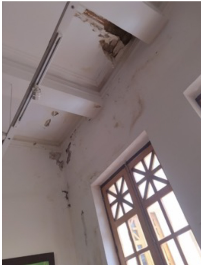
Figure 9. Moisture Due to Water Infiltration
