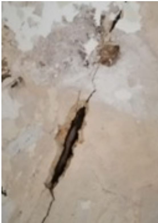
Figure 11. Crack Due to Settlement
