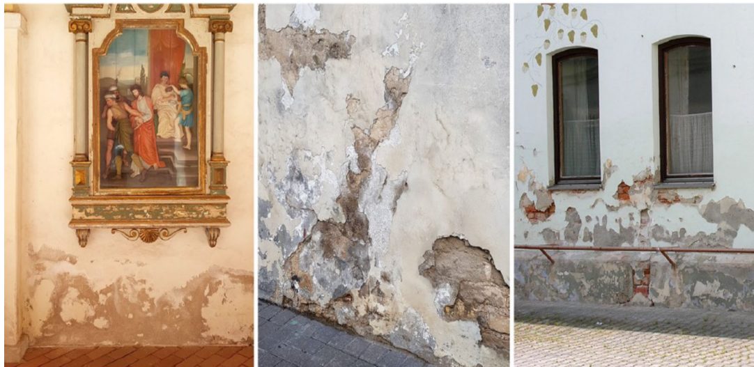
Figure 2. Examples of Salt Weathering and Moisture-Related Decay in Brick Masonry Substrates: (a) Poland; (b) Latvia; (c) Germany [11]
