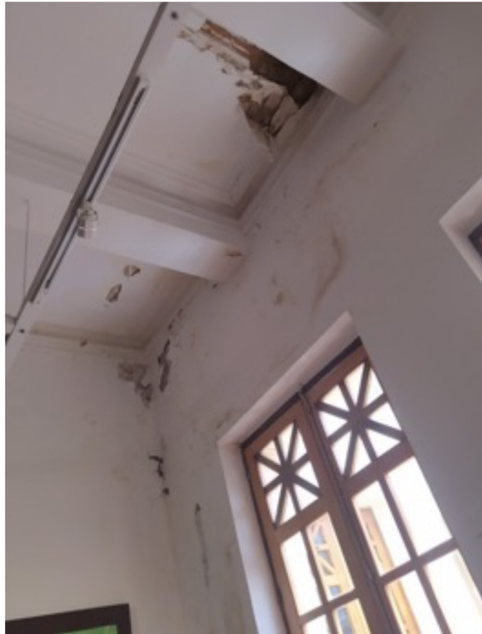
Figure 9. Moisture Due to Water Infiltration
