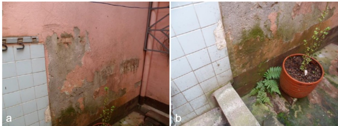
Figure 5. (a) Efflorescence and Mortar Cracking; (b) Bulging and Cracking of the Plaster [29]
