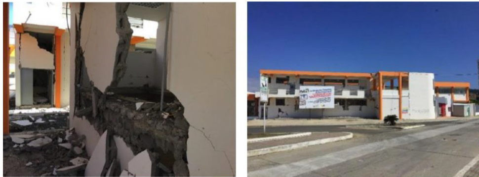
Figure 4. Structural Failure of an Educational Facility Induced by the April 2016 Seismic Event [6]
