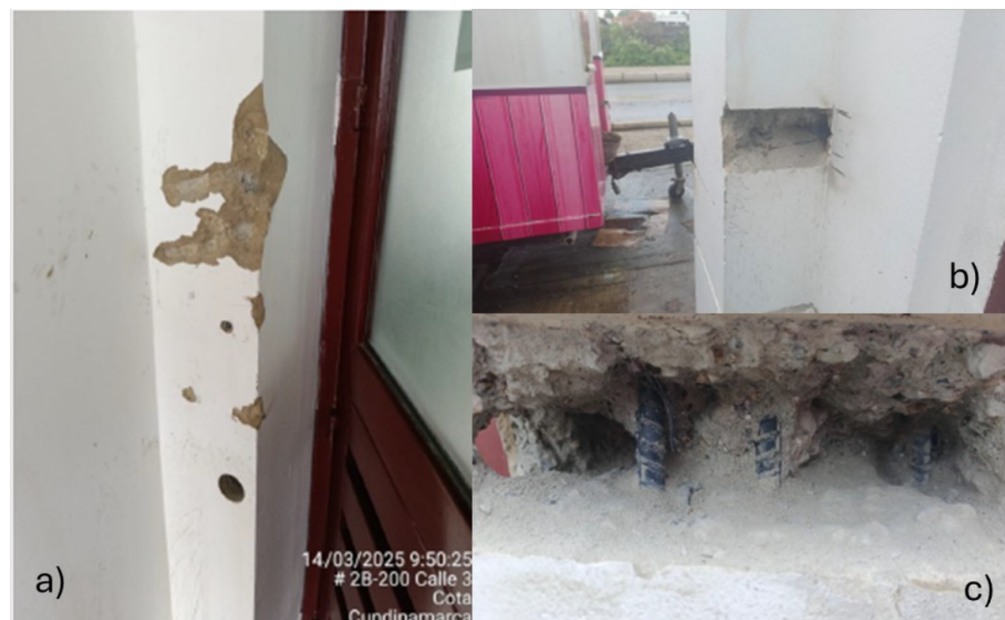
Figure 7. a) Corner, b) Pitting, and c) Pitting Without Corrosion
